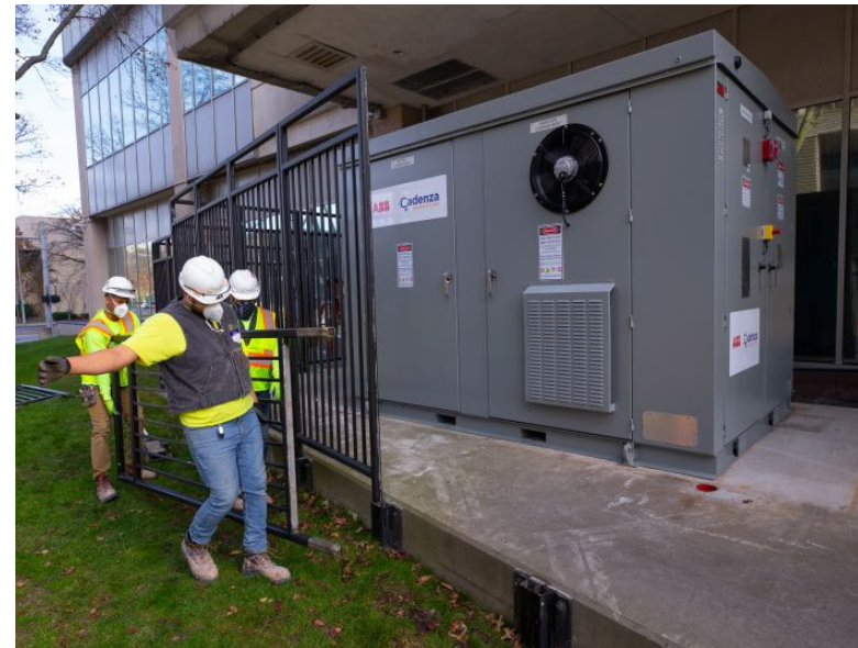
Small Commercial – 250 kWh
