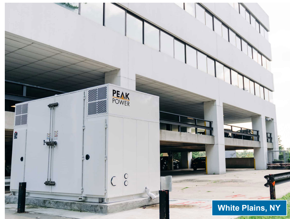
375 kW / 940 kWh installation: Commercial project at office park in Westchester County.
