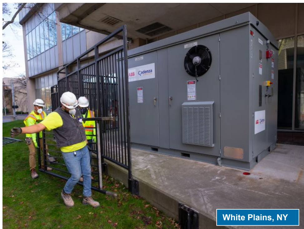
50 kW / 250 kWh installation: Commercial project at NYPA HQ in Westchester County.
