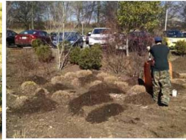
Figure 17. Mulch replacement is one activity that may be included in a maintenance agreement for stormwater practices such as bioretention.
