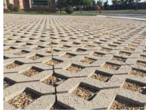
Figure 5. Concrete grid pavers are a good option to reduce runoff from parking lots
